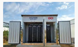
300kWh commercial ESS at the OCI Plant
